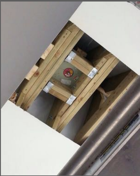
Image left is the Winch concealed in the loft above the ceiling and Image right is the Overboarded Ceiling
